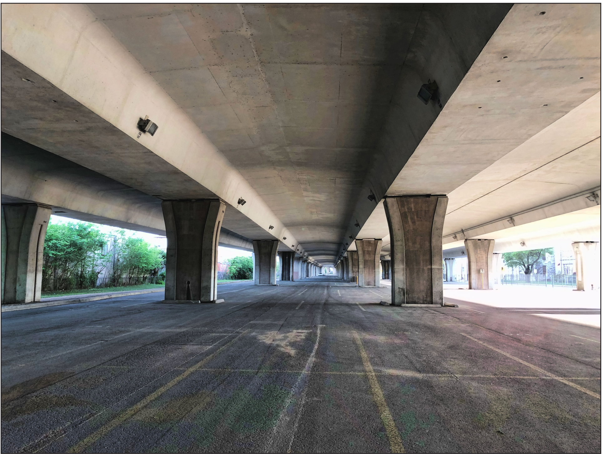
[Figure 22] - Underpass Lighting - Existing
